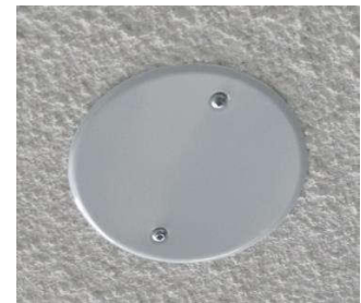
Ceiling Electrical Box
