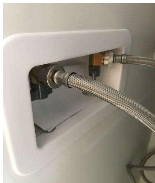
Water Shut-Off Valve
